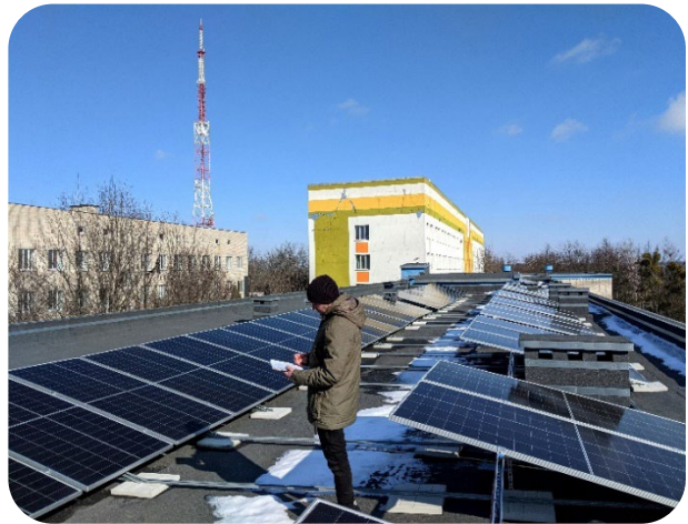
PV panels at the roof of the hospital
