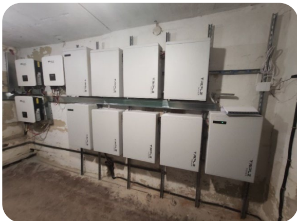
Batteries and controllers of the PV station in the basement
