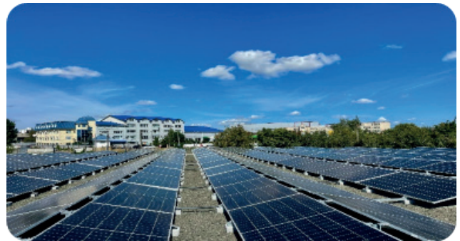
PV panels at Lutskvodokanal's buildings
