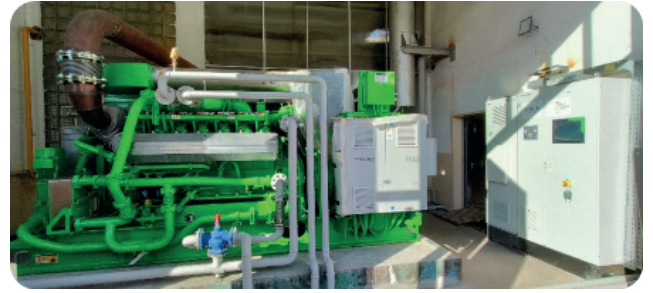
CHPs in a boiler house in Khmelnytskyi
